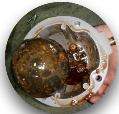
Mixed lubricated oil pollutants inside the drain body
